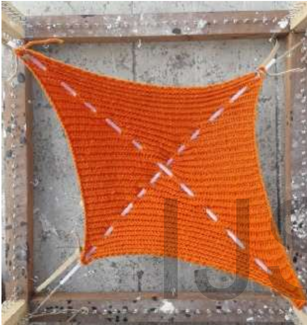
Fig. 72 Plan View Prestressed knitted cloth as stay in place formwork Prestressed knitted cloth as stay in place formwork
